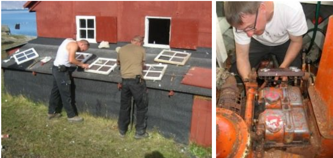
Left: Repairation of Ørnereden's window. Right: Per prepares the engine in "Agsut".
